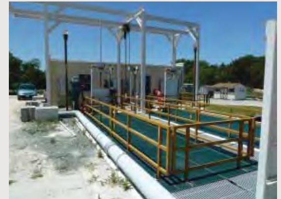
1. Water Pump Station
