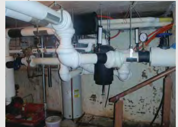
2. Geothermal system at Center Administration
