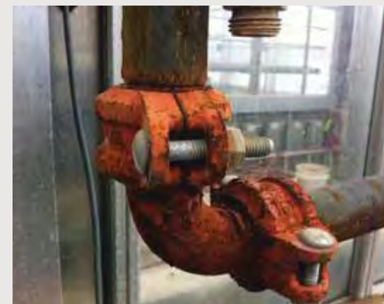
3. AL Greenhouse - Deteriorating plumbing system
